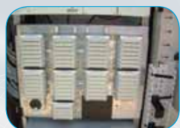
DS1 Compact Blocks for OSP Cabinets
